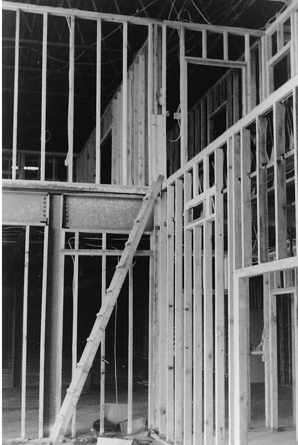
Fig. 12.1.11 A view of framing for the first- and second-story offices of a plant, with a roof beam and the steelwork supporting the second floor visible. (Source: VMA, Inc.)
